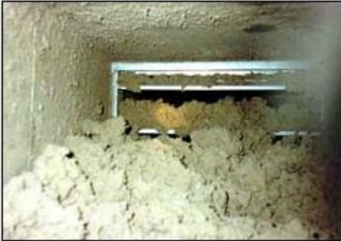
clogged air ducts can be a health hazard...
